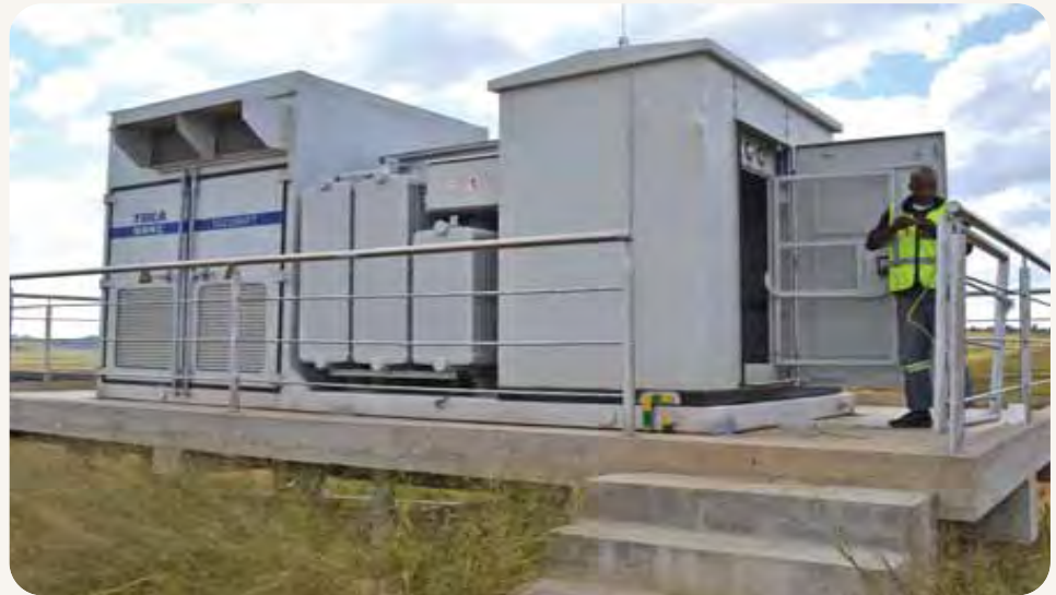
One of the inverters at at Ramarothole solar Power Plant used to convert direct current from a network of solar panels to alternating current for home use
