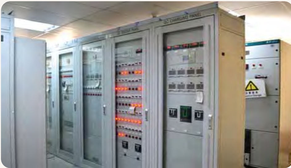
Controls and monitors used at Ramarothole Station
