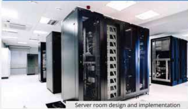
Server room design and implementation
