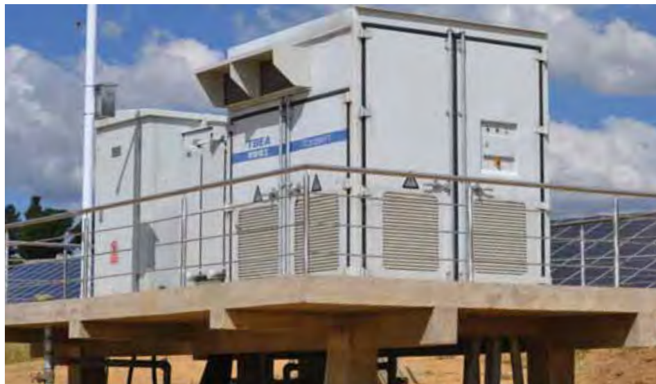
Giant inverters convert direct current to alternating current used in the grid
