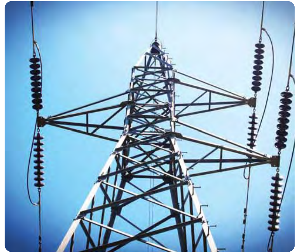
High voltage power transmission lines
