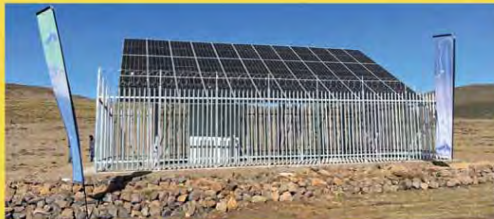
Solar Power Plant at Sani Border Post
